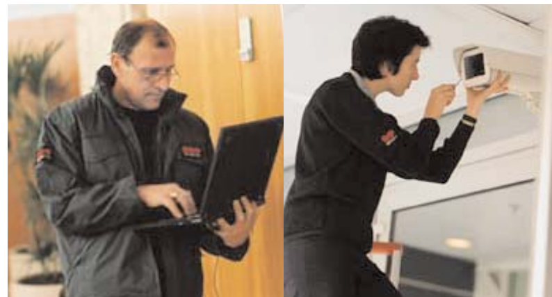
Roger Raillia is a technician for Security Systems Paris. The division last year equipped over 800 BNP Paribas branches with additional electronic systems (CCTV+ alarms). Caroline Ducoin, Branch Manager, Security Systems Paris, carrying out maintenance on a client's security camera.
